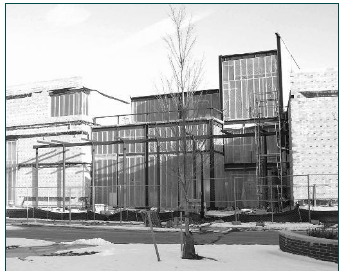
The new Plainsboro Library takes shape at the Village Center. The project is on schedule for construction to be completed this summer.
