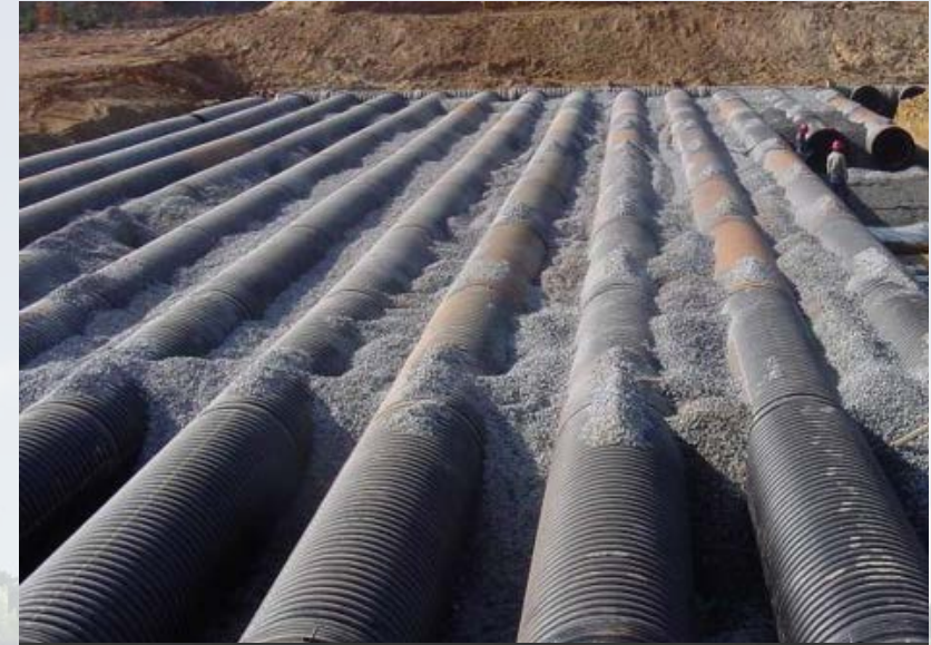
Underground Retention System
